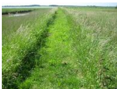
7 Area of path (in foreground) that over topped in 2007 surge tide. (Close to the pump station)
