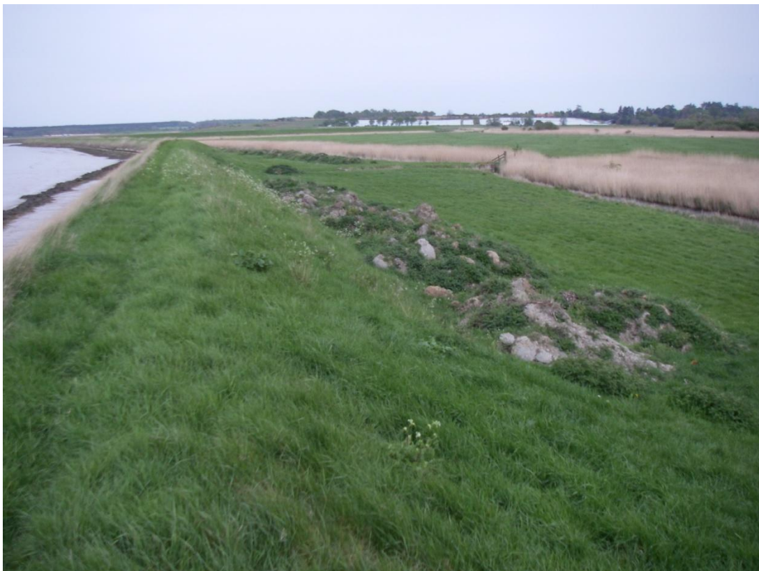
View looking north from Ch 750m, steep angle of landward wall to be reduced. Landowner is drying fill for this purpose.
