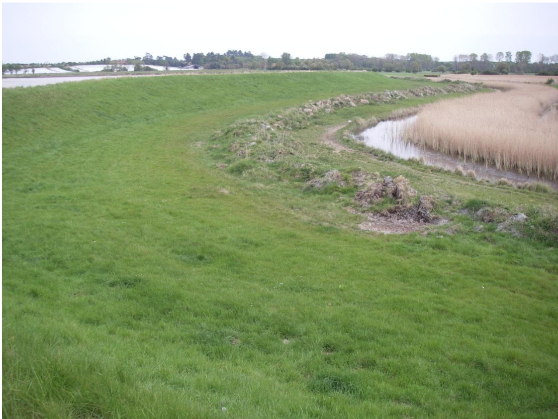
View from Ch 1020m looking north, note drying borrow material and space to borrow ditch.
