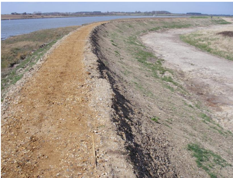
View looking west from Ch 1500. High and steep landward slope requiring three anchor rows.
