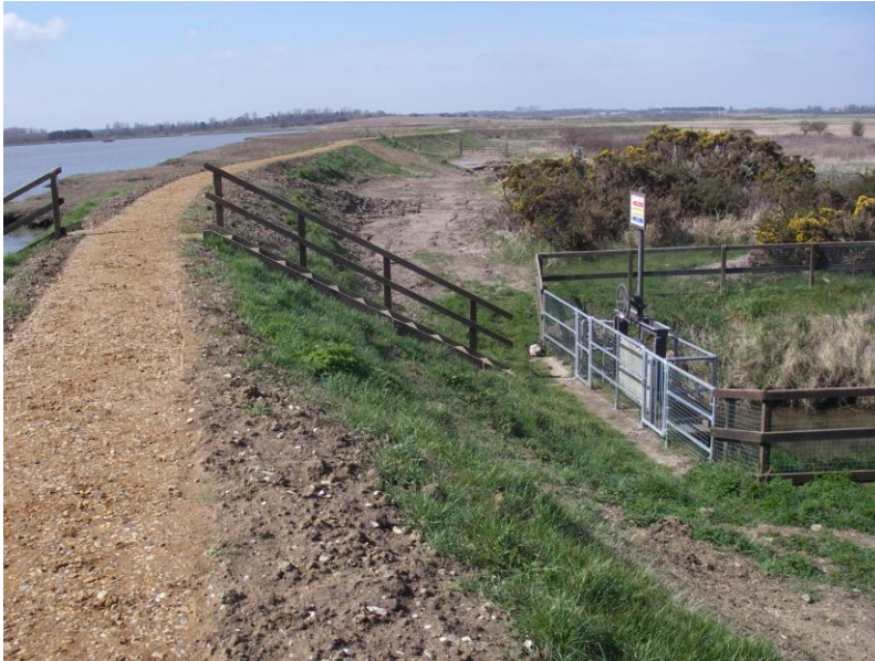
View looking south west from Ch 650. Slacket landward slope requiring only two anchor rows.
